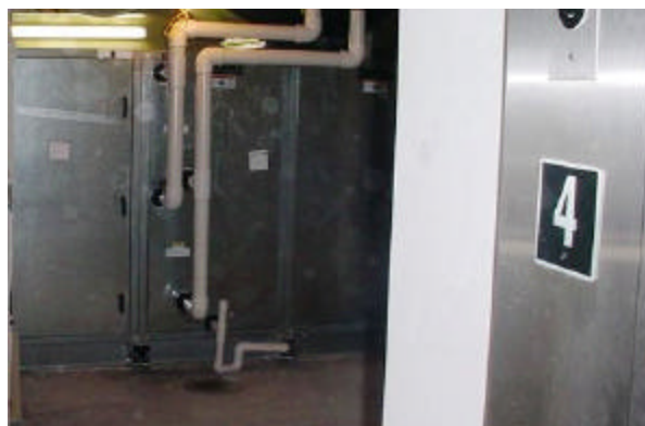
New air handlers on 4 th and 3 rd floors have been swapped out
